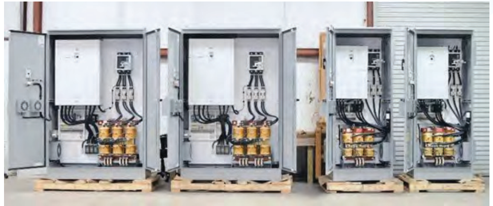
400HP & 150HP AS100CP Clean Power VFD's
